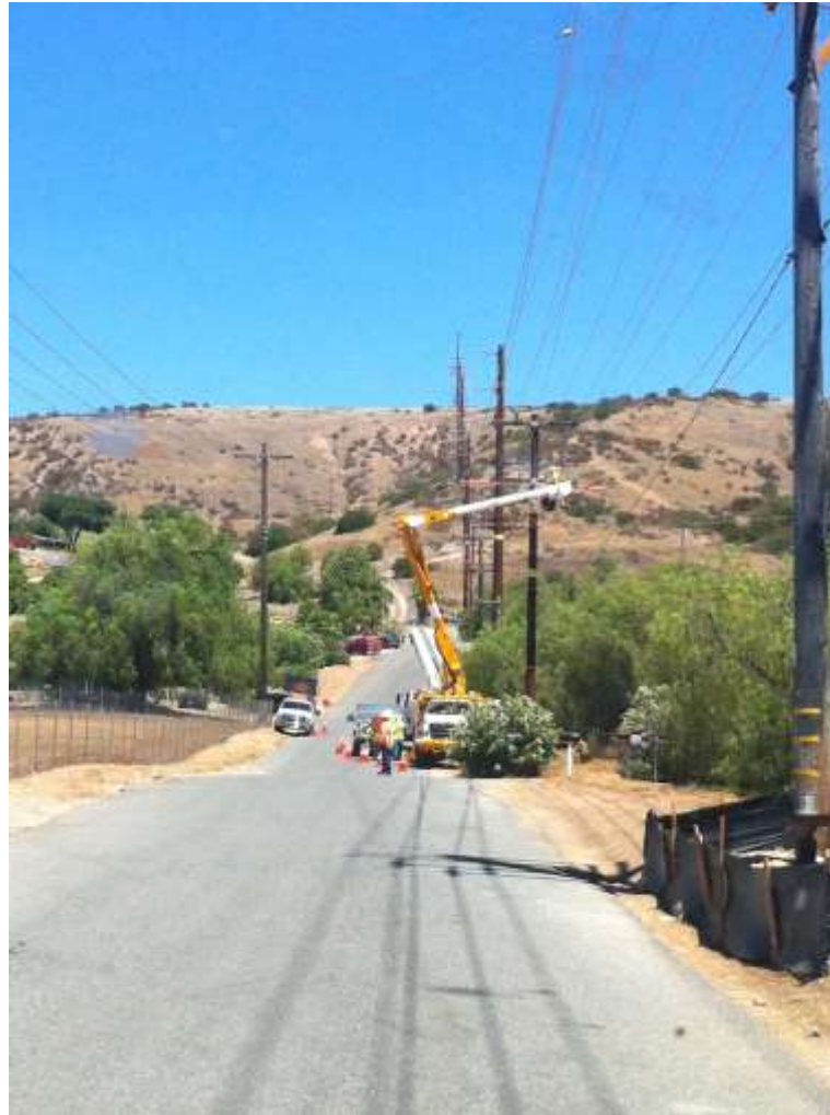
Photo 1: Construction crews were observed conducting overhead wire activities along Creelman Lane, which included installing in-line disconnects (pictured above). Traffic control measures including signage, flags, cones and traffic directors were implemented around work areas in accordance with APM TRA-1.
